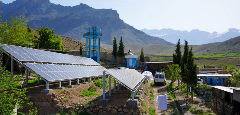
A solar-powered water system at a Kisaw District Hospital in Daikudi, Afghanistan, built with support from UK aid. © UNICEF/UNI981283/Fazel
